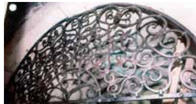
4 Projekt 2: stanje rešetke nakon čišćenja Project 2: condition of metal grating after cleaning
