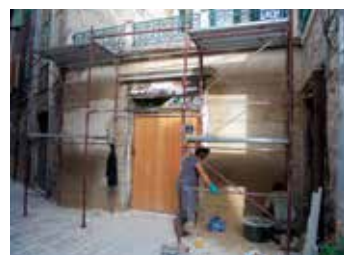
36 Projekt 45: stanje uličnog zida u tijeku radova Project 45: condition of street wall during restoration
