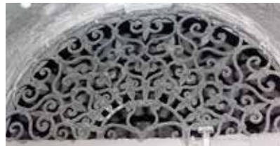
3 Projekt 2: stanje rešetke prije radova Project 2: condition of metal grating before restoration
