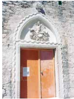
18 Projekt 19: stanje portala neposredno nakon intervencija Project 19: condition of portal immediately after restoration
